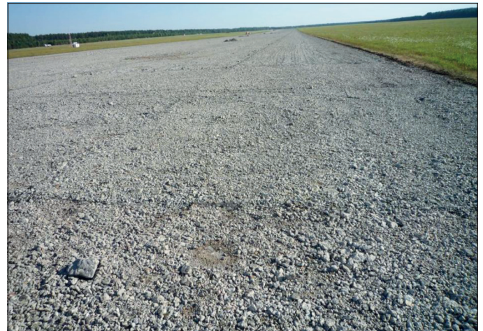
Fig. 19. Broken pavement; photo by the author
