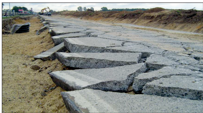
Fig. 1. Broken pavement slabs in the A18 highway; photo by the author
