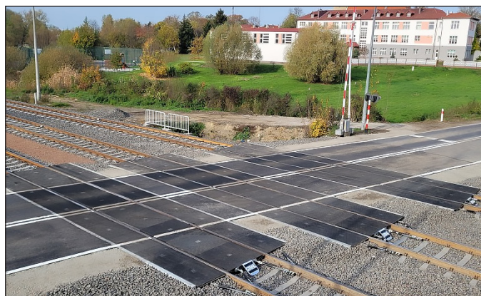
Fig. 3. Railway level crossing with an automatic user-side protection (category B) with pavement made of rubber crossing slabs
